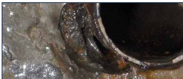
Hole at the Tube to Tubesheet Interface
