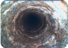
Condenser Tube After Metal Scraper
