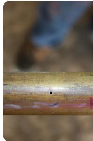
Condenser tube w/ pinhole
